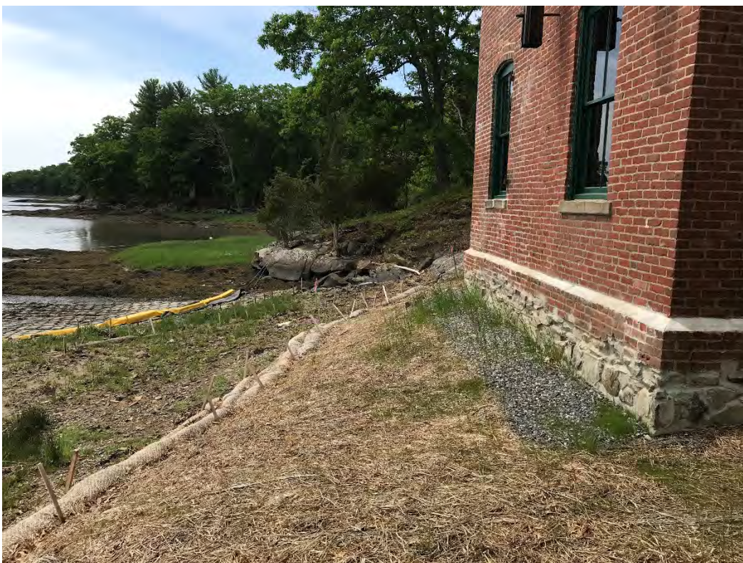
Fig 2: Slope between the cable house and salt marsh restoration at the west side of the bay. Viewing south. (06-01-21)
