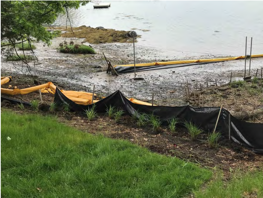
Fig 11: Plugs installed at the toe of slope at Gundalow Landing/east side of the bay. Viewing south. (06-01-21)
