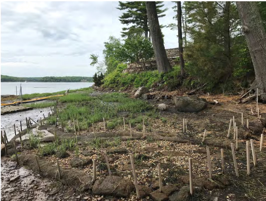
Fig 12: Salt marsh restoration at Gundalow Landing/east side of the bay. Viewing northwest. (06-01-21)
