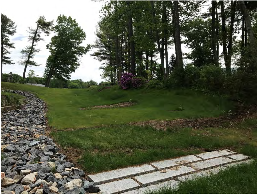
Fig 9: Slope above the manhole at Gundalow Landing/east side of the bay. Viewing east. (06-01-21)
